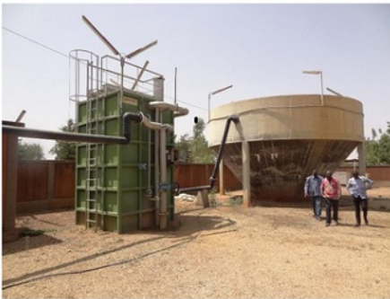
ONEA treatment plant in Boromo
